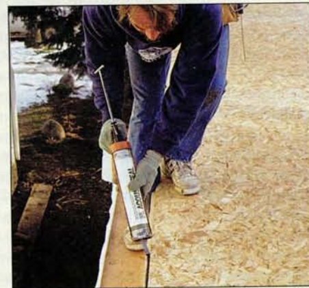
Second-floor rim-joist seal. To provide an air barrier at second-floor rim joists, Tyvek strips are sealed with acoustical caulk to top and bottom wall plates. Here, David Schuman puts a bead of acoustical caulk along the wall before it's raised into place.
